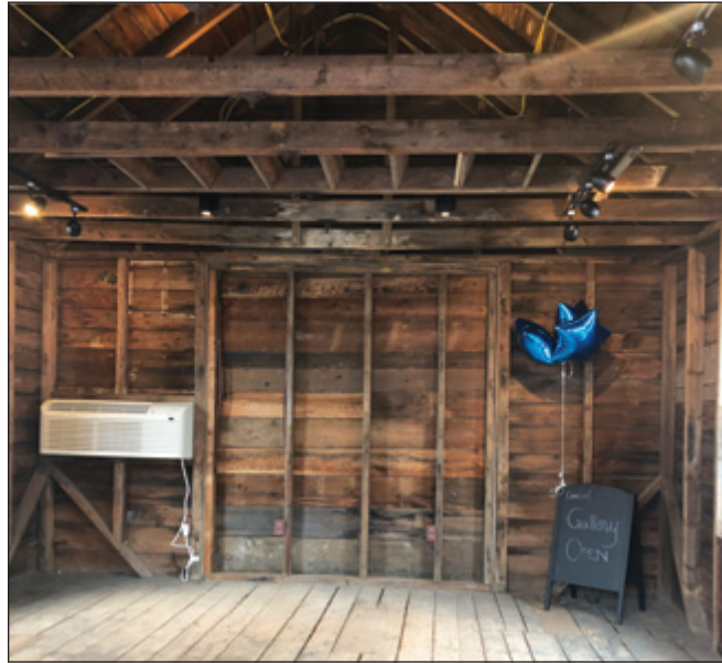
The Concept Shed at Millbrook Station offers temporary space for all kinds of businesses.
